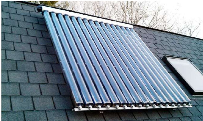
Figure 2.5: A rooftop solar thermal array for domestic water heating.
