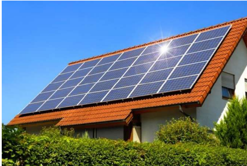
Figure 2.2: A rooftop array of photovoltaic cells.
